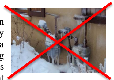
Frozen Meters & Regulators due to water from upper deck
